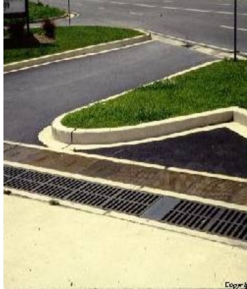
Figure PTP-01- 6 Perimeter Sand Filter
