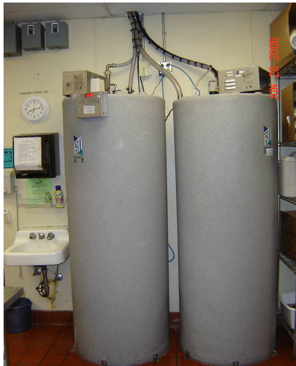
Figure PTP-07- 2 Internal Grease Collection System
